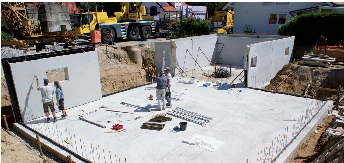
Construction site White tanks: Application wolfseal KB Elements as well as FTS Elements
